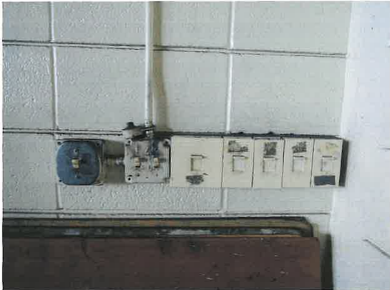
q. Evidence of intrusive modern technology. post-dating electricity Terminus Post Quem = 1800s
